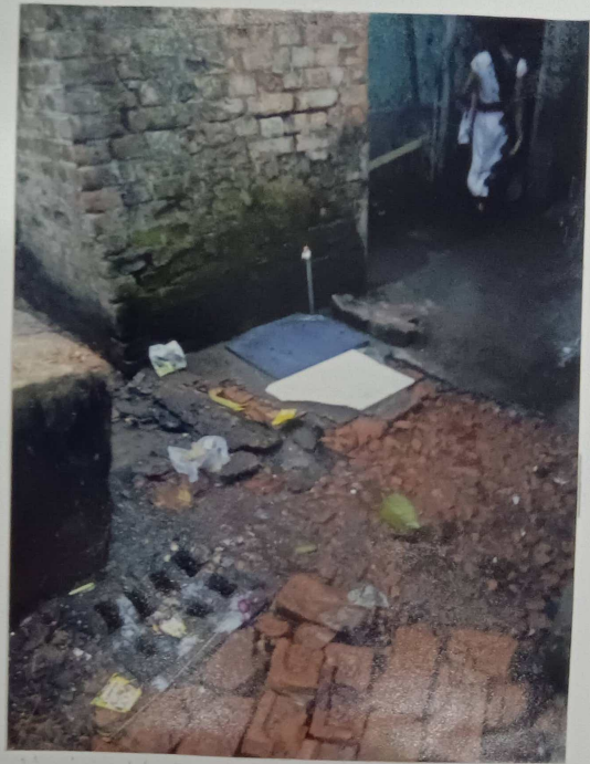
MUNICIPALITY TAP WATER LOCATED NEAR A DRAIN
